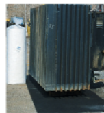
Ideal underneath leaking transformers.
